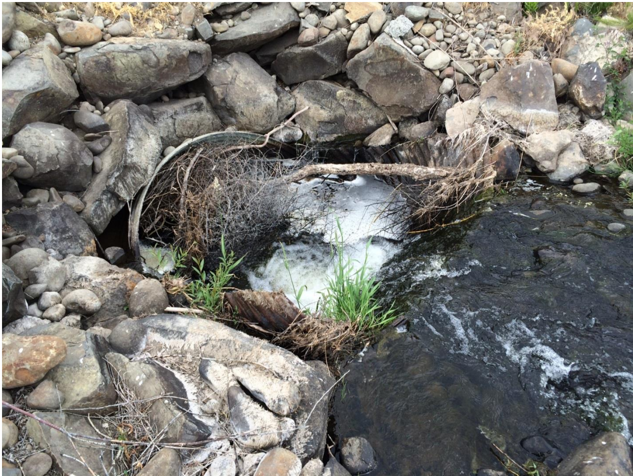
Figure 8. The entrance to the Town Canal undershot appears susceptible to plugging due to debris or ice however its performance is will be a key factor in controlling the level of flooding on the Woods property. The ability to perform maintenance on the entrance during a large flood is questionable.
